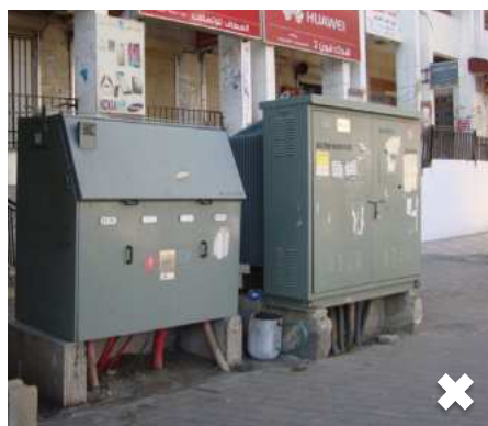
Exposed utilities on sidewalk
