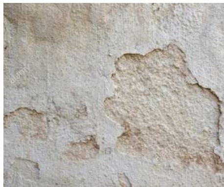
Poorly plastered surface
